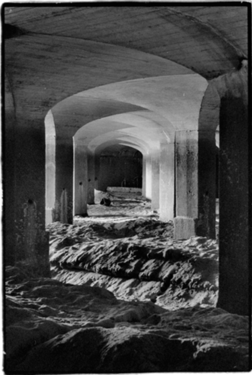
Cover: Lincoln Memorial, looking down from memorial attic space. Above: Disused water filtration plant. Right: St Elizabeths Mental Hospital, historic west campus.
