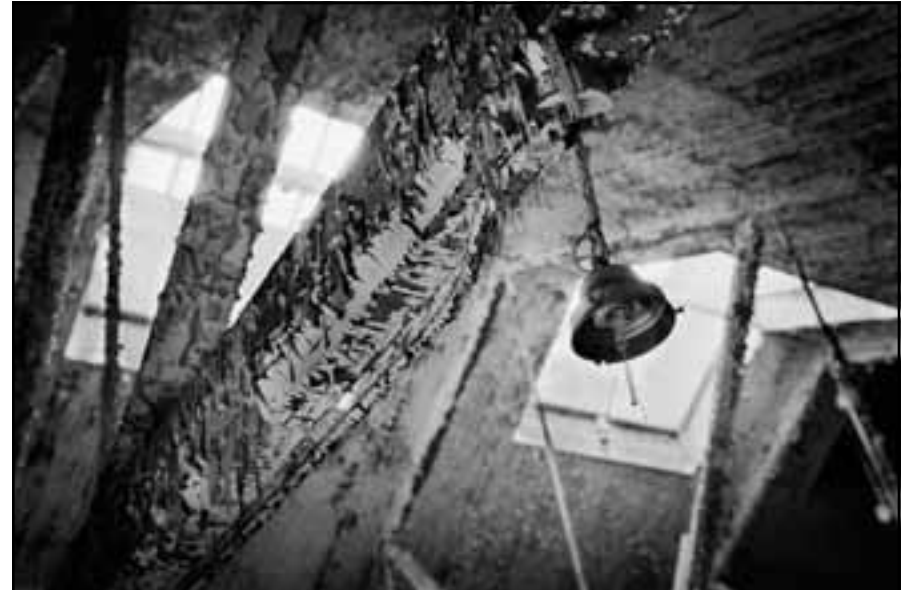
Peeling paint and fixtures at disused bakery.
