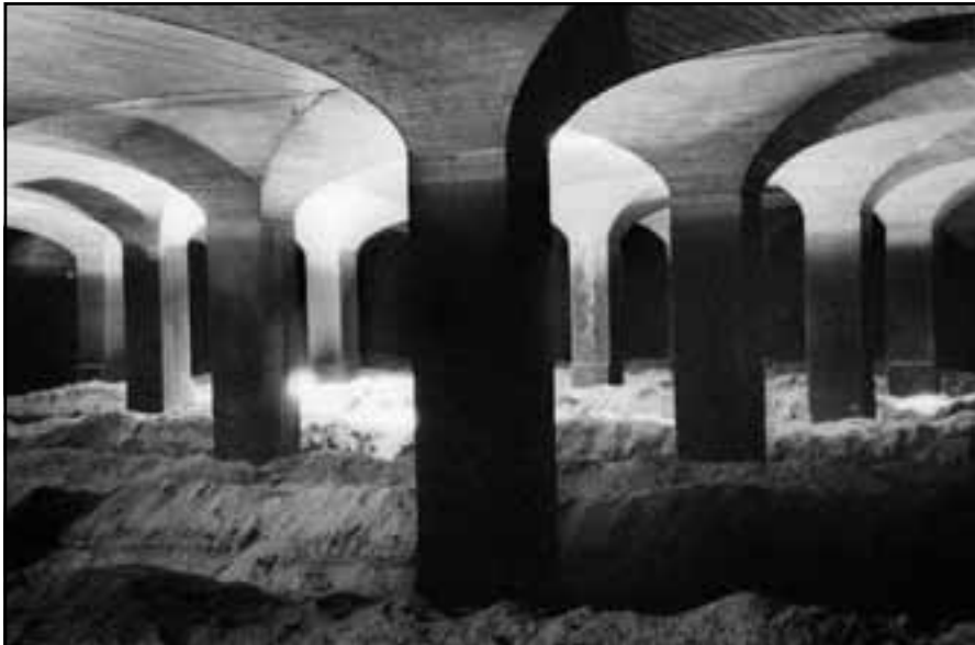
Water Filtration Plant
